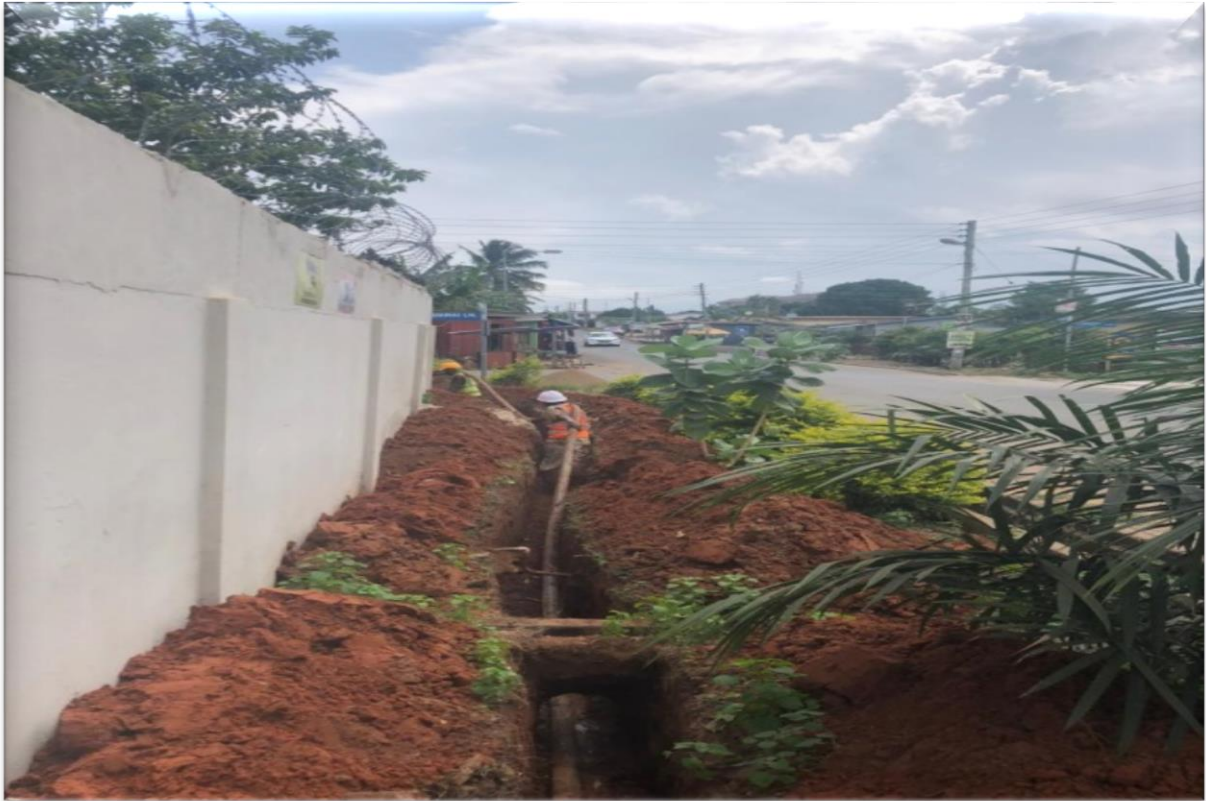
Laying of Under Ground Cable at Mukose Street – MiDA Project (Kaneshie District)
