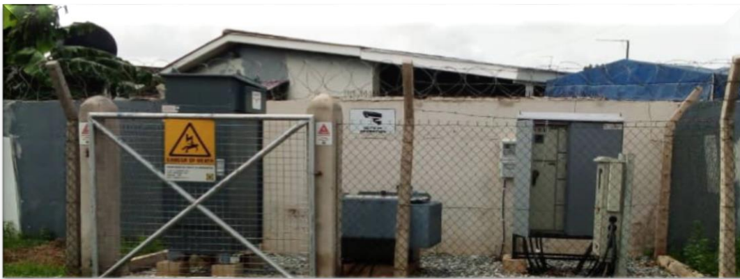
Fencing, completion and commissioned of GMT Substation at Mukose Street – MiDA Project (Kaneshie District)
