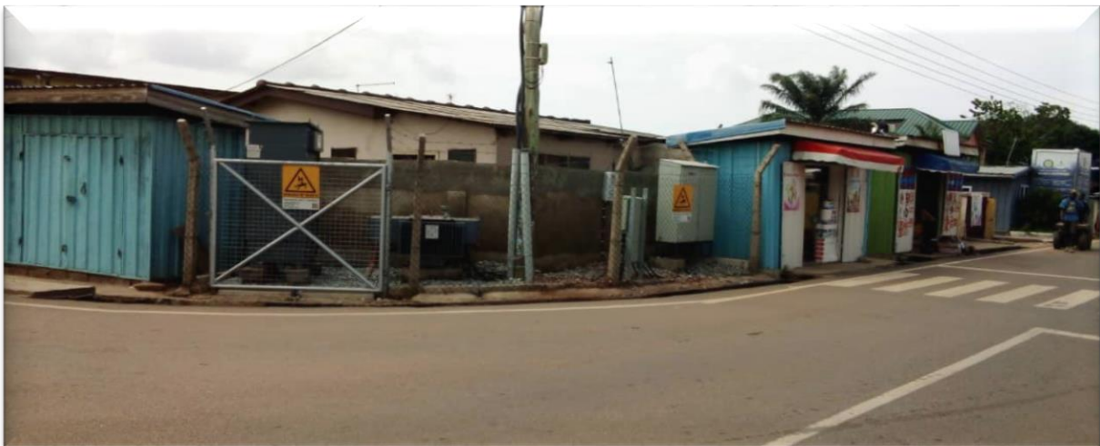
GMT (200KVA TX, RMU and DP) substation completed and commissioned at Swanlake North Kaneshie
