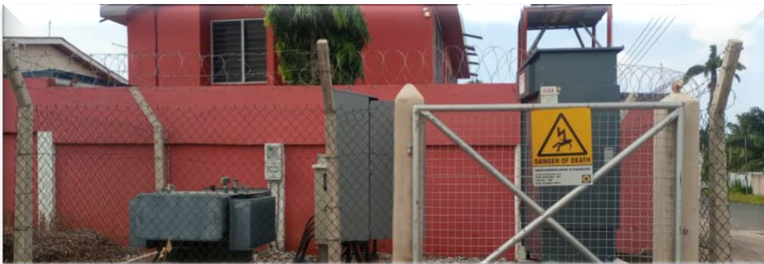
Concrete Plinth for GMT Substation Foundation works and completion of GMT substation at SS Omane Street – MiDA Project (Kaneshie District)
