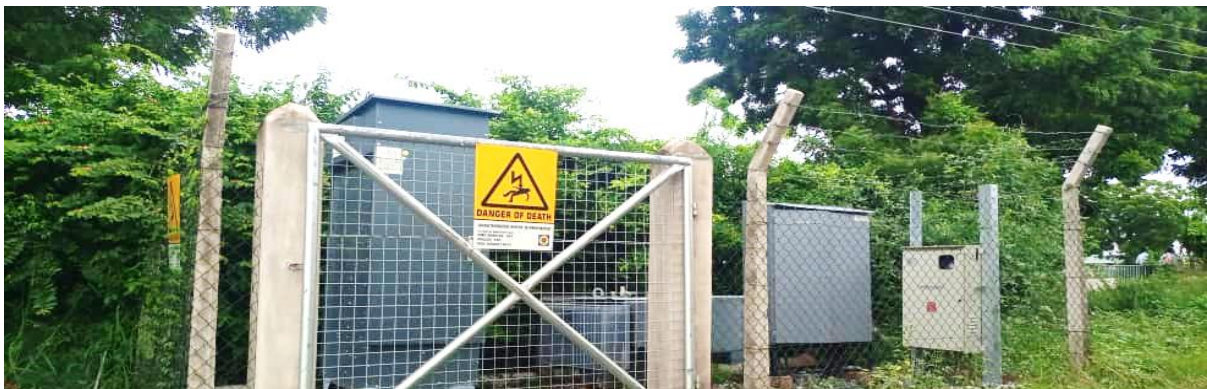
GMT Substation completed and commissioned at the Ghana Police Training School, Accra - MiDA Project (Under ECG Kaneshie District)
