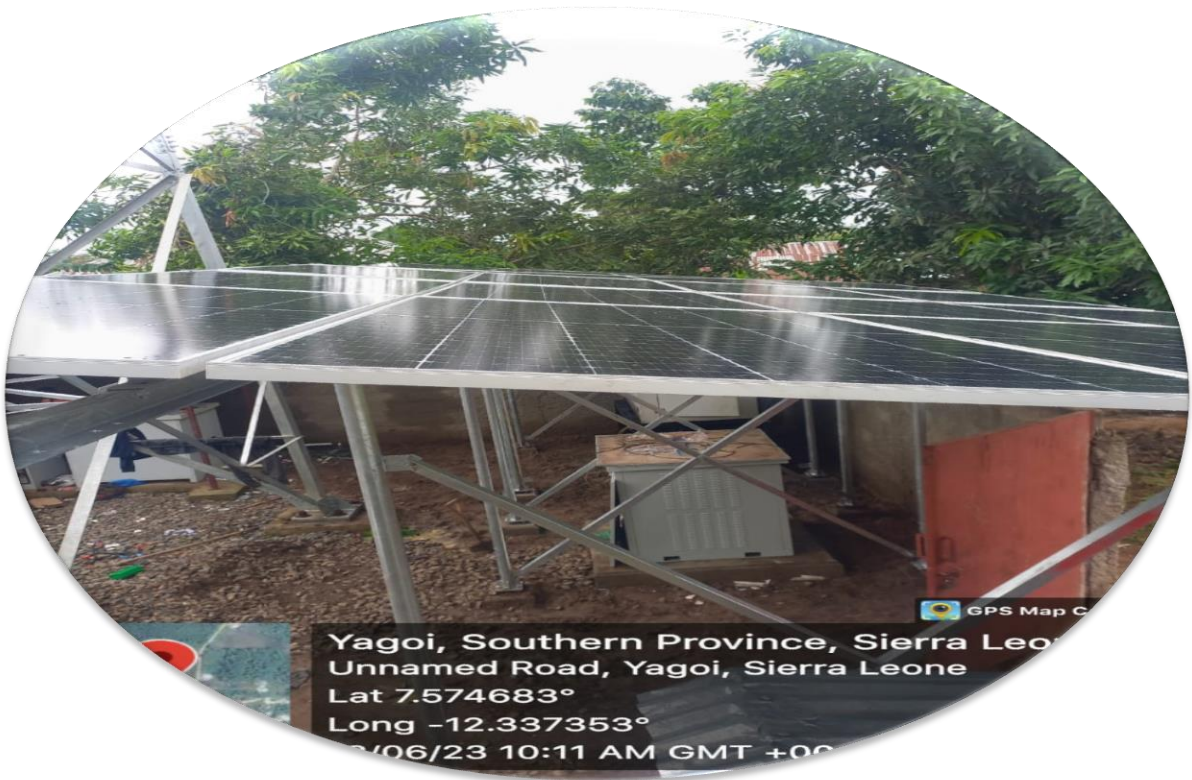
PV Solar Installation works completed at Rokupr and Yagoi Qcell site in Sierra Leone by GP Solar Team
