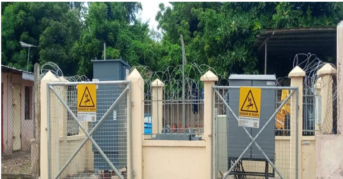
Mounting of RMU, DP and 200KVA Transformer , completion and commissioned of GMT at AwudomeCemetary – MiDA Project (Kaneshie District)
