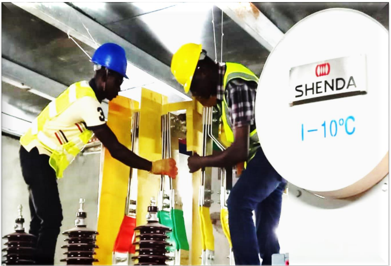
Installation of Busbars arrangements on 4MVA Transformer to the DP by Gross Pool Engineering Team at Yunzu Fiber Factory
