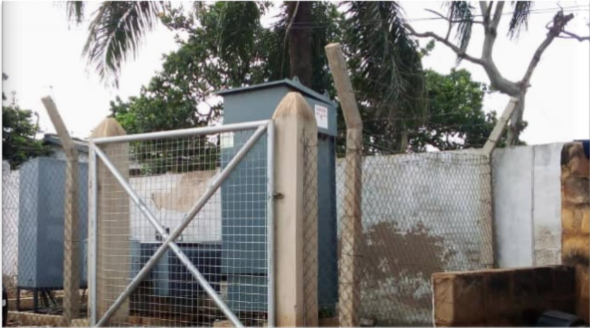
GMT Substation Foundation works, mounting of RMU, DP, 200KVA Transformer fully completed and commissioned at Cable & Wireless – MiDA Project (Under ECG Kaneshie District)
