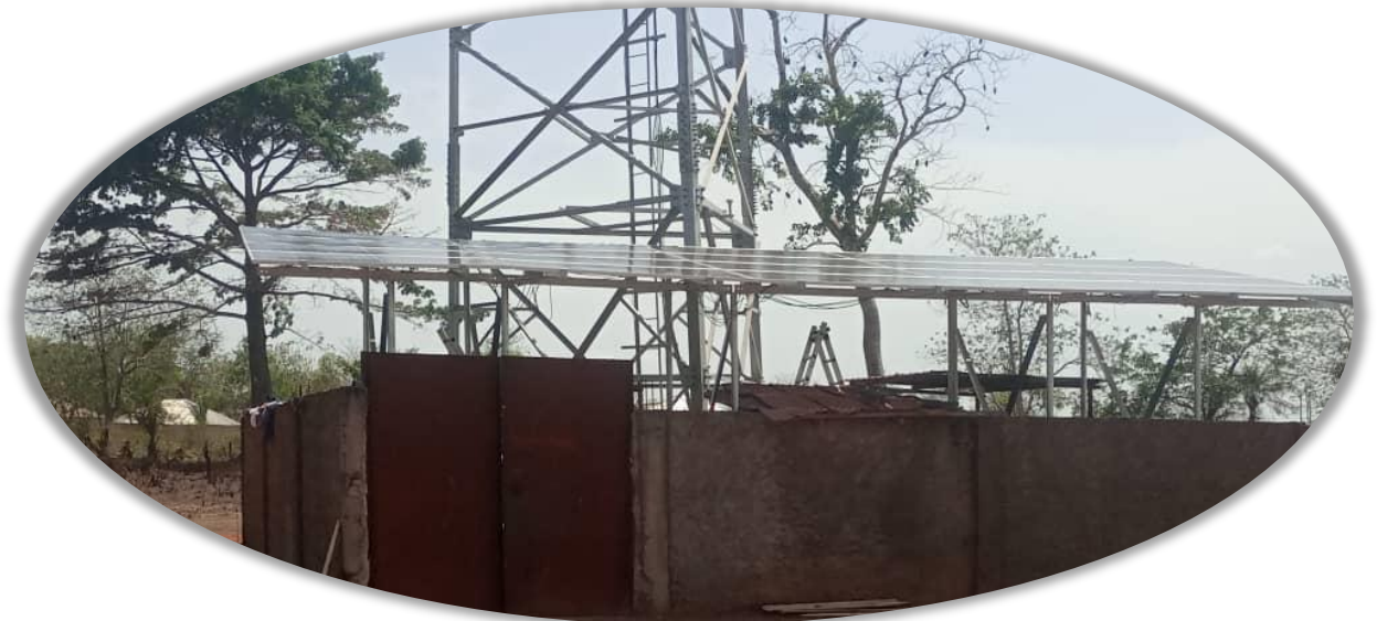
PV Solar Installation works completed by Gross Pool Engineering Solar Team in Sierra Leone for Qcell site
