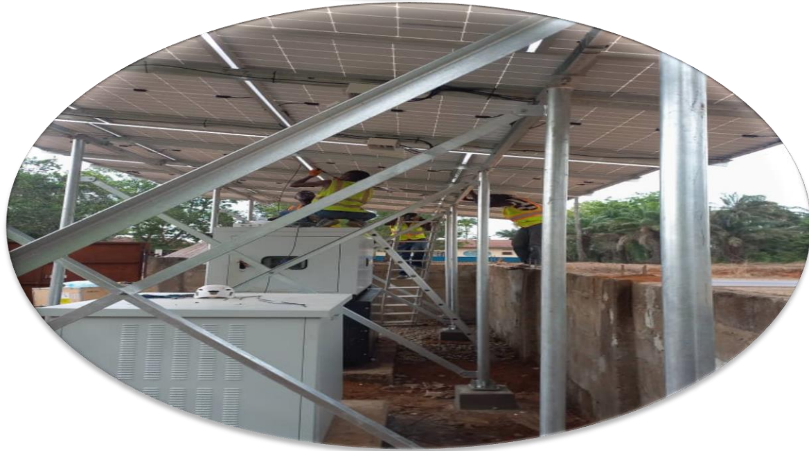
Gross Pool Engineering Ltd, Our Solar Team on Installation of PV Solar System and Battery Bank at QCELL Site Near Port Loko in Sierra Leone (May, 2023)
