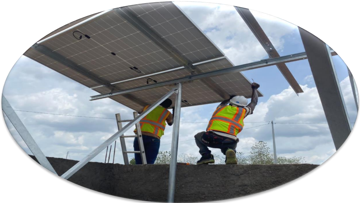
Gross Pool Engineering Solar Team at work in Sierra Leone at Qcell Site
