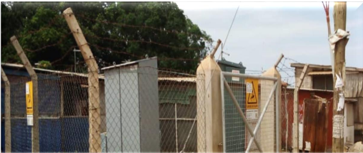
Final fencing and GMT Substation completed behind Accra Academy School – MiDA Project (Kaneshie District)
