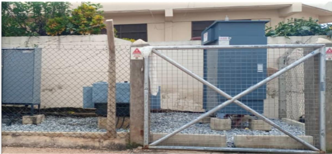
Fully completed and commissioned GMT Substation at Abeka Market down – MiDA Project (Kaneshie District)
