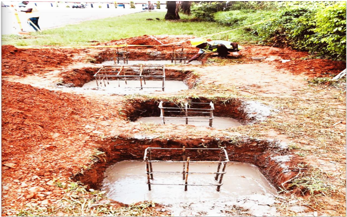
GMT Substation foundation works at the Ghana Police Training School, Accra - MiDA Project (Under ECG Kaneshie District)
