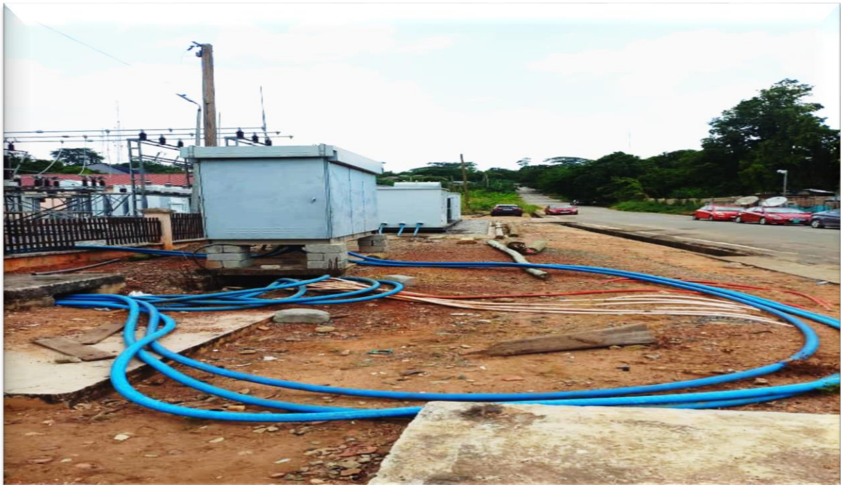
Laying of 1X630sqmm UG Cable to be connected to the main Feeder at the Nsawam ECG Substation
