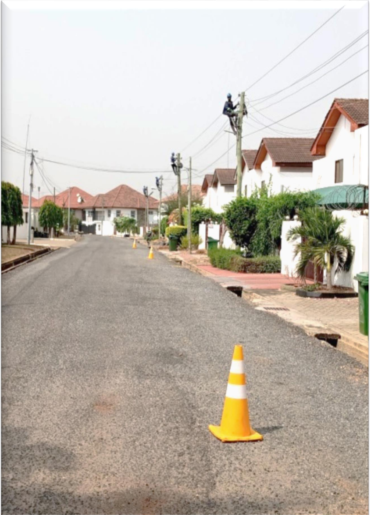
LV Network Improvement at NTHC Estate Adjiringanor East Legon – MiDA Project (Undr ECG Legon District)
