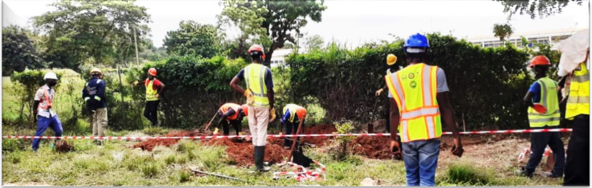
Getting the ground prepared for the construction of GMT Substation at the Ghana Police Training School, Accra
