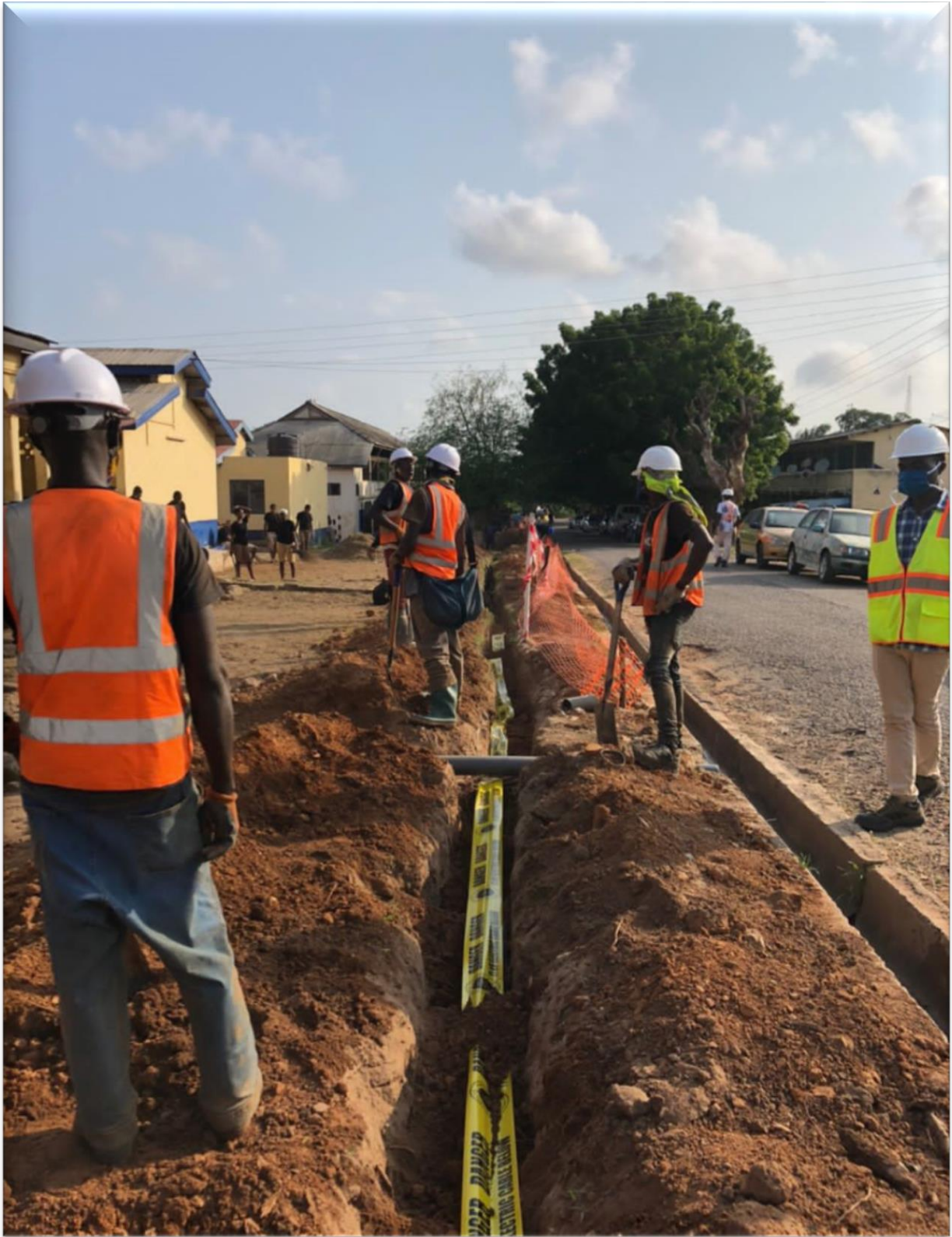
Laying of Under Ground Cable at Police Training School Accra – MiDA Project (Kaneshie District)
