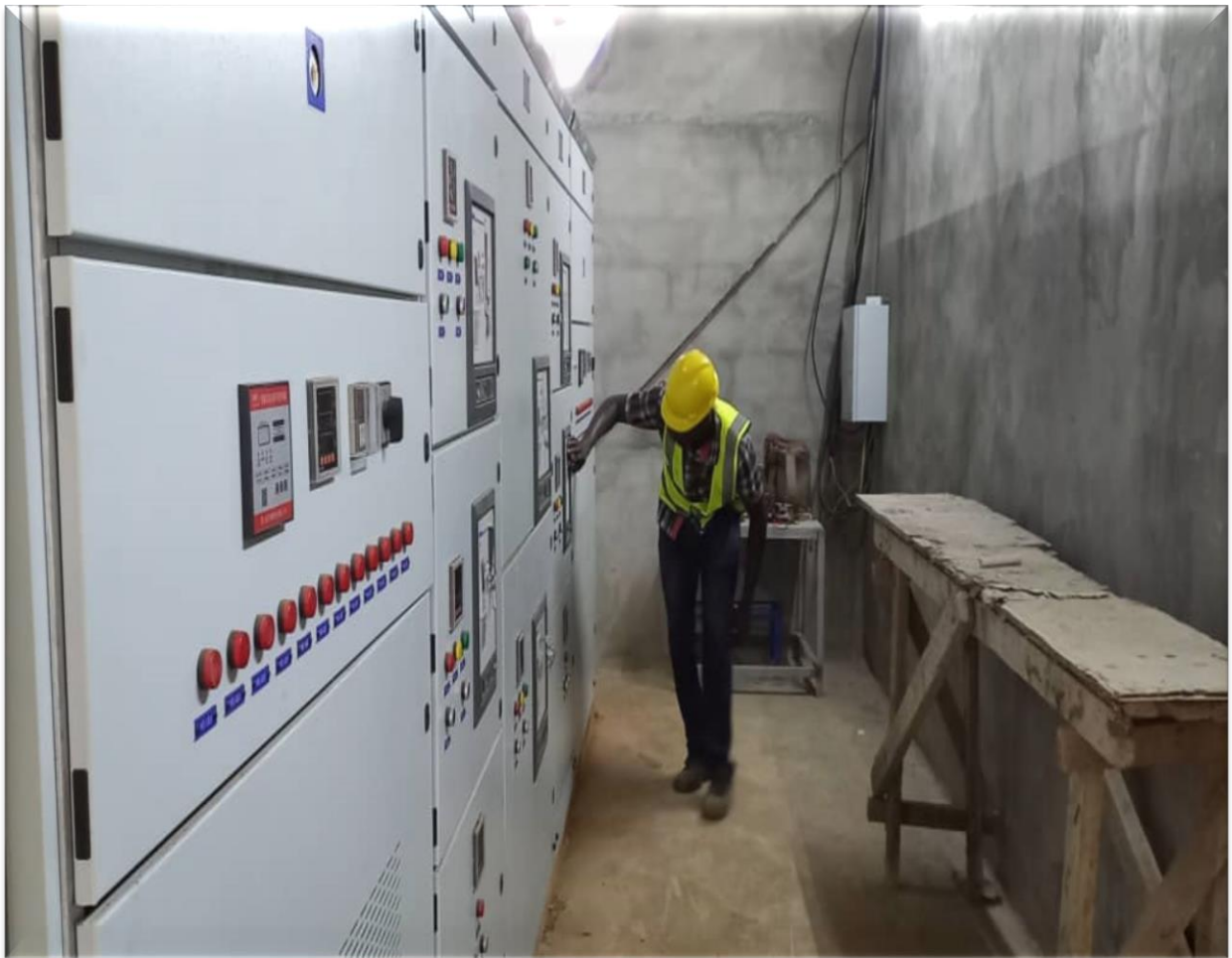
Finalizing on DP arrangement and Termination at the Yunzu Fiber Factory Substation
